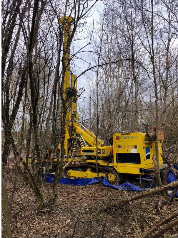
FIG. 8. Photo of the ongoing drilling of a core at the proposed FPF location to assess the geological conditions.
